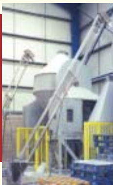
Mobile conveyors feeding cone blender.
