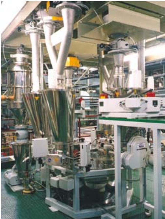
Modular volumetric and loss-in-weight feeders integrated with a gravimetric blending system and K-Tron PCS loaders in a plastics extrusion process
